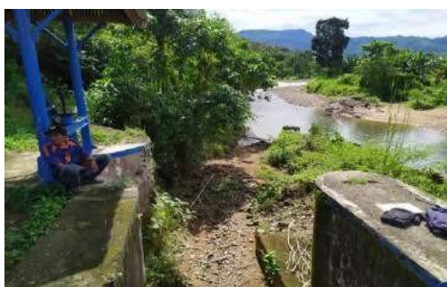
Figure 15. Kasang II Dam covered by sediment
