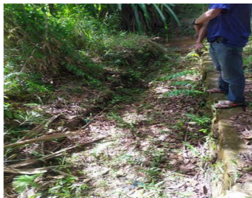
Figure 3. Damaged Kapalo Hilalang canal.
